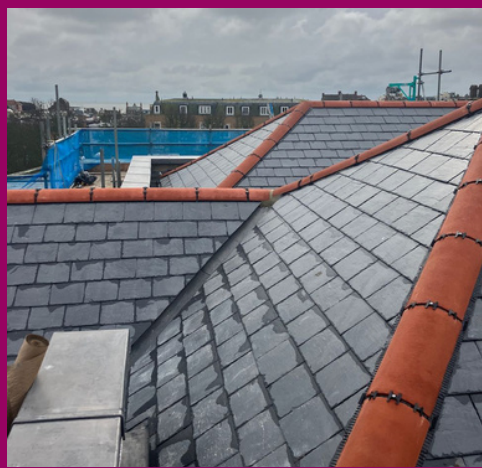
Work was completed on a new roof and toilets at our listed building, Foresters Hall, thanks to funding from the Colyer Fergusson Charitable Trust.
